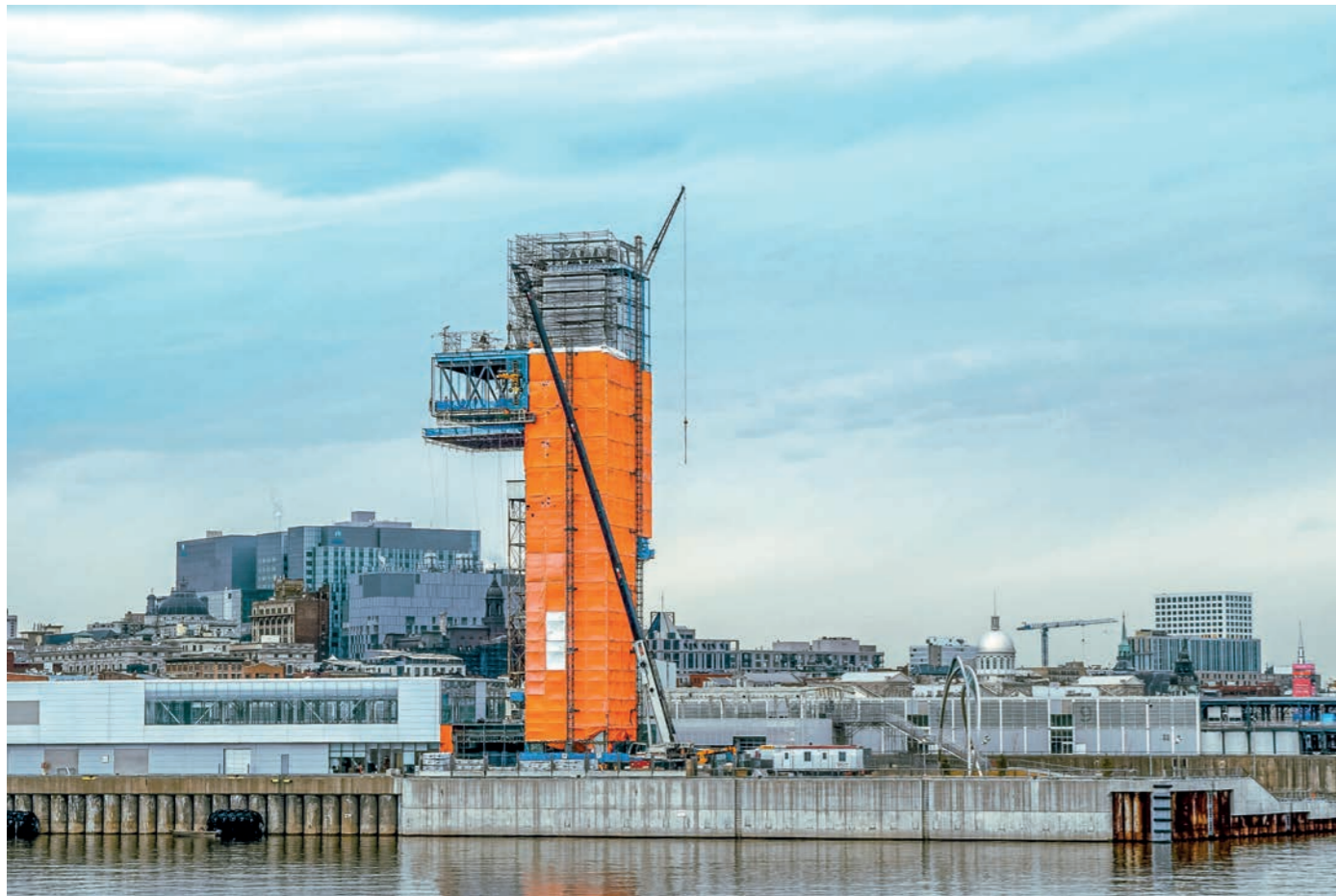
Montarea sticlei Heavydrive la Tour du Grand Quai din Montréal QC (Canada)
